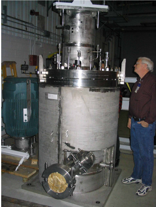
External View of Pump
