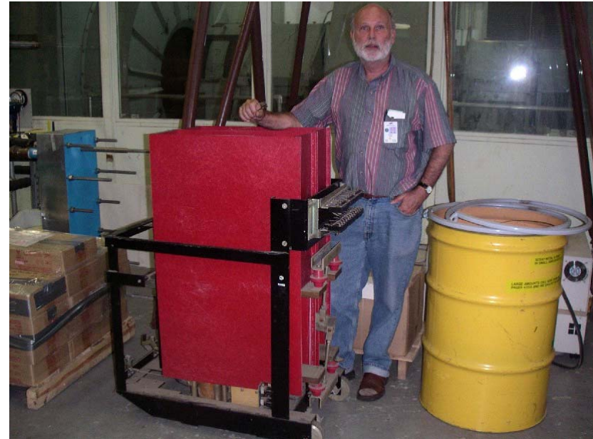
Mechanical switch for 4.4 MW
