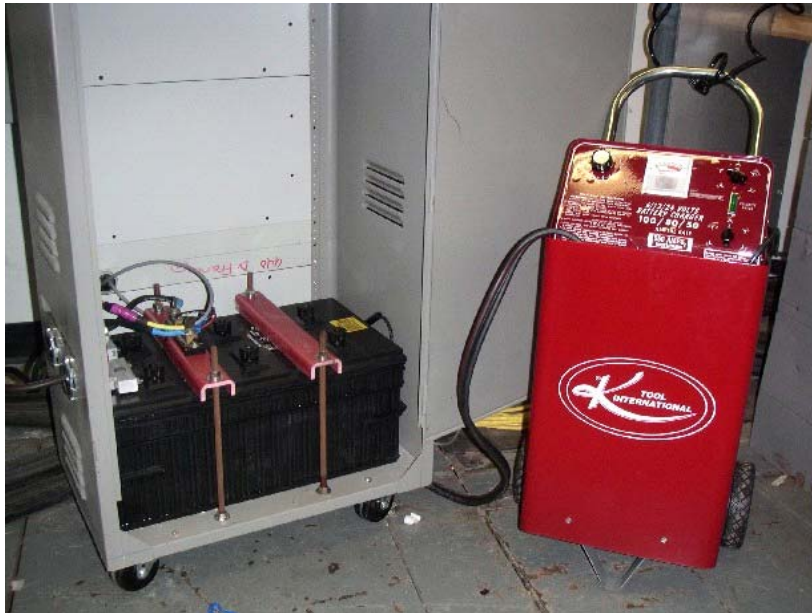
Battery and charger (12 V, 1400 A)
